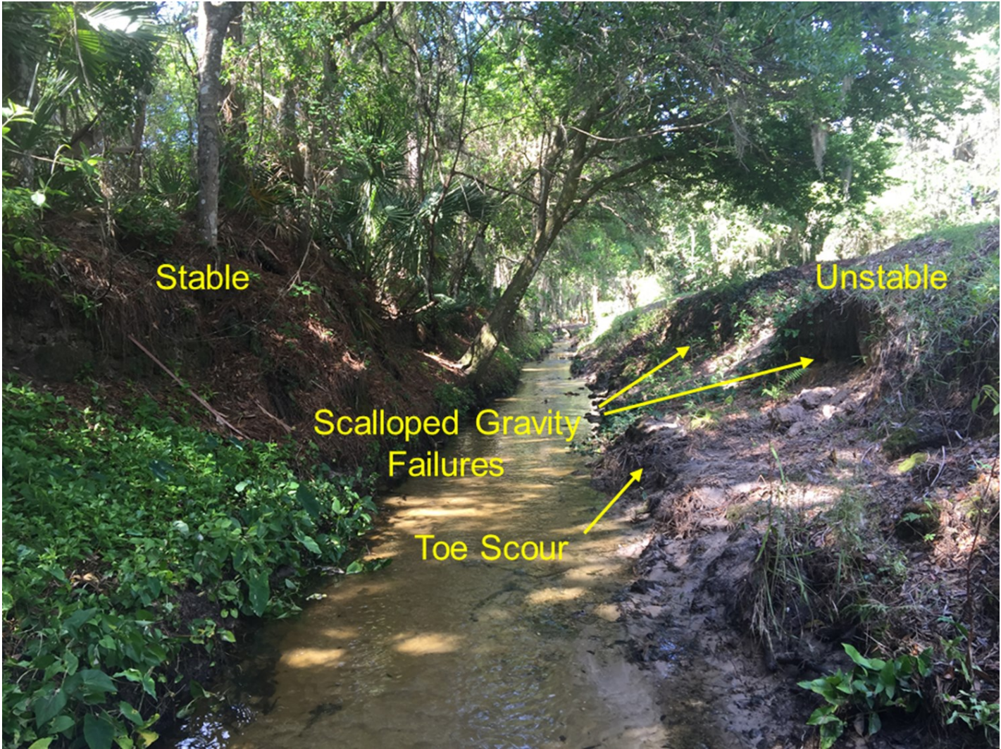
The canal in the example above is in the early stages of evolving into a more stable two-stage channel, with a small floodplain (bankfull bench) being carved out between the toe scour and scalloped gravity failures on the grassed right bank. If left untreated, erosion will destroy the travelway above it and will deliver many tons of sediment downstream over a period of several decades. In contrast, the left bank is forested and resisting erosion.
