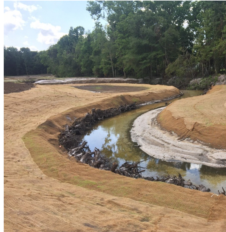
Rosgen Toe Wood. A cantilevered log and stump array that stabilizes bends and sustains deep pools with fish habitat akin to an overhanging bank.
