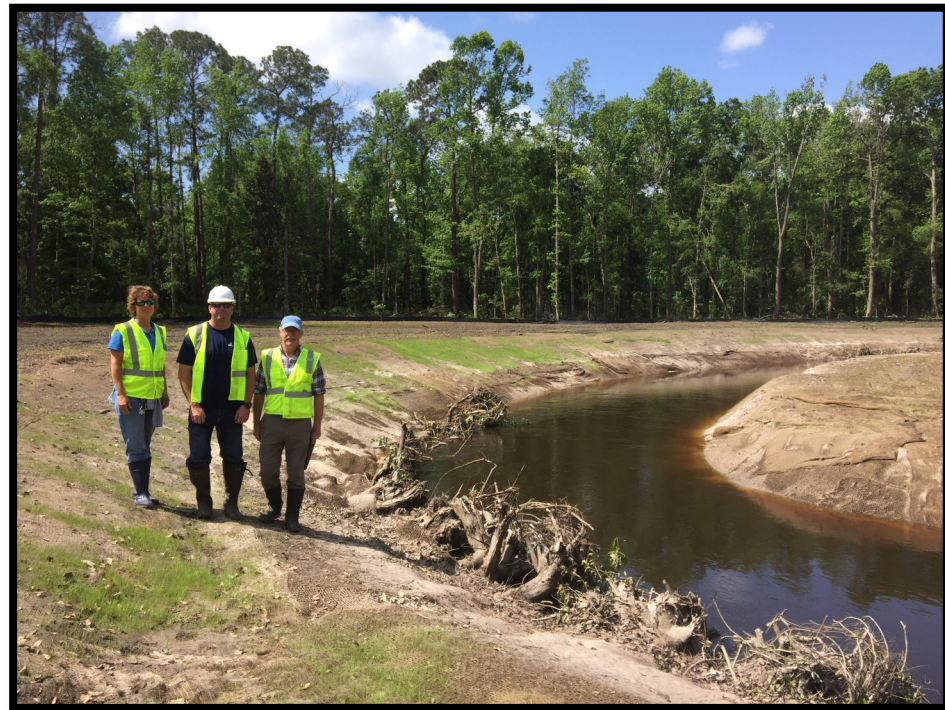
Sarasota County staff visiting the Suwannee River Water Management District’s conversion of the Alligator Creek canal to a natural channel in Starke, FL. Wood designed the project to be fully funded by the Florida Department of Transportation and Florida Fish and Wildlife Conservation Commission. A variety of game fish built spawning beds in the restored stream habitat within a year of project construction. Spawning was concurrently absent in the canal immediately upstream and downstream of the project.
