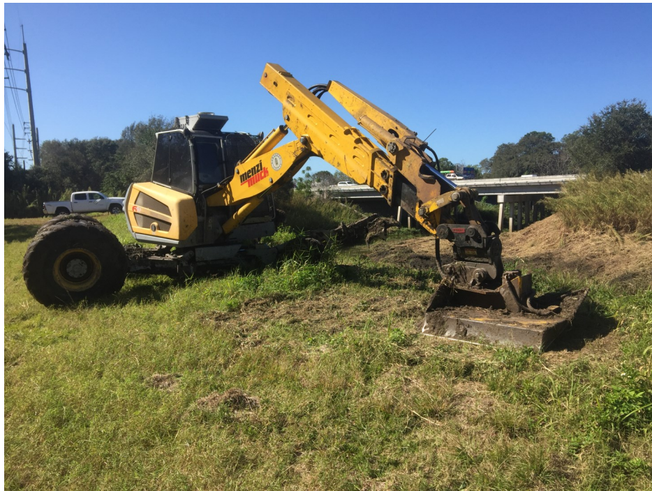
Skilled operators use the County's walking excavators to climb in and out of the canals to remove sediments and debris and mow brush on the banks. These specialized waterway maintenance machines can work on steep slopes and in up to several feet of water.
