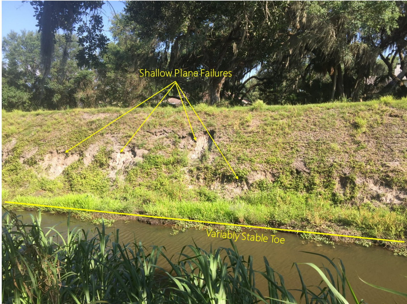
The canal in the image above has banks in excess of 15 feet high at a side steeper than 2:1 (H:V—horizontal:vertical). Shallow rooted grasses simply cannot hold the sandy bank materials together with such severe morphology absent frequent repairs.
